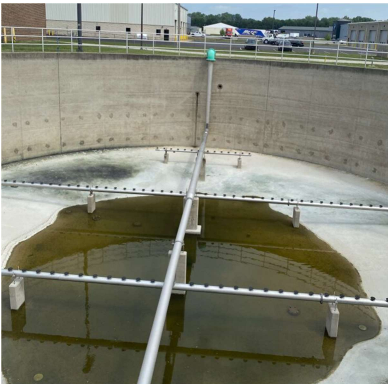
Figure 4-14 Inside of an Aerobic Digester
