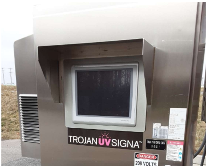
Figure 5-3 Existing UV Control Panel
