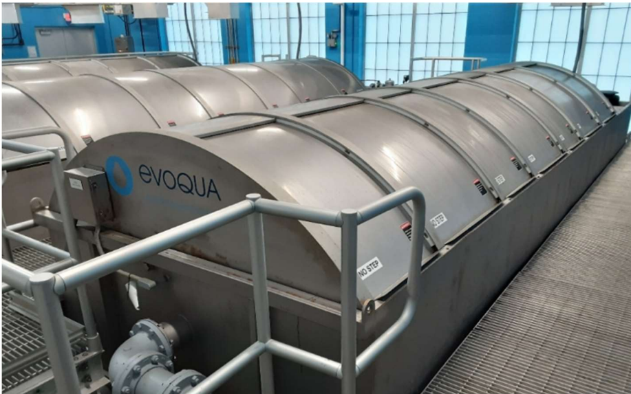
Figure 4-11 Existing Evoqua Filters
