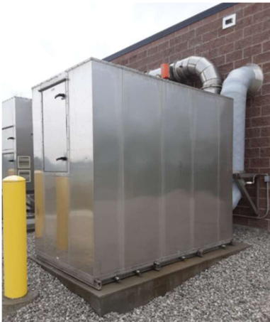
Figure 5-9 Existing Odor Control Equipment
