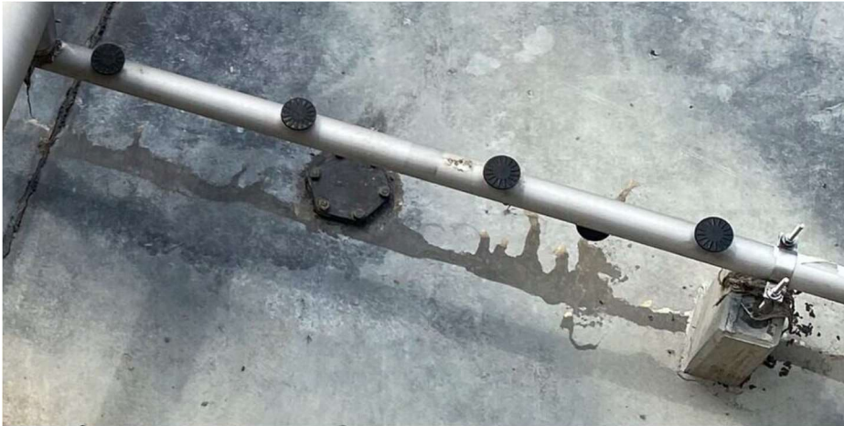
Figure 5-13 Existing Digester Diffusers
