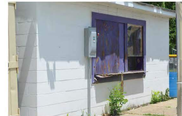
Outbuildings / Various Levels of Disrepair
