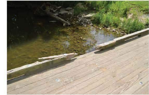
East Ped Bridge / Damaged Protective Barrier
