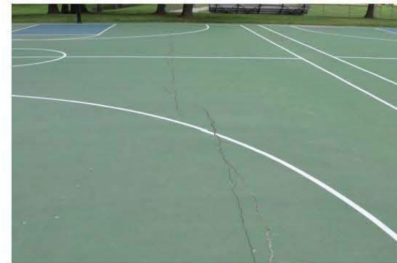
Basketball Courts / Surfacing & Cracking
