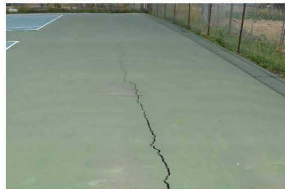
Tennis Courts / Surfacing & Cracking
