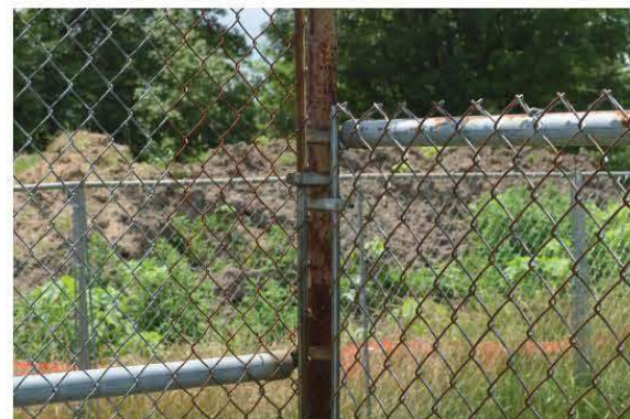
Fencing / Various Condition Issues
