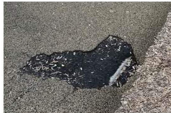
Blast Off / Various Surfacing & ADA Shortfalls
