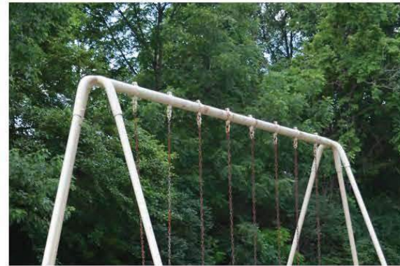
Playground / Various Condition Issues
