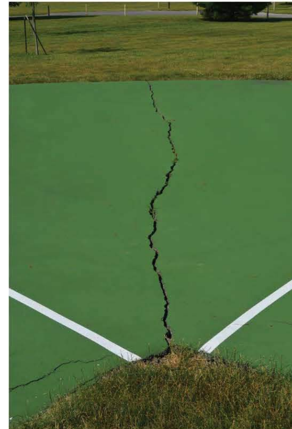
Basketball Courts / Subsurface Issues
