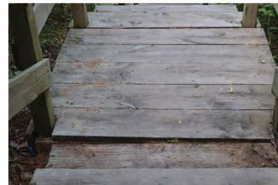
Pavilion Stairway / Trip Hazards
